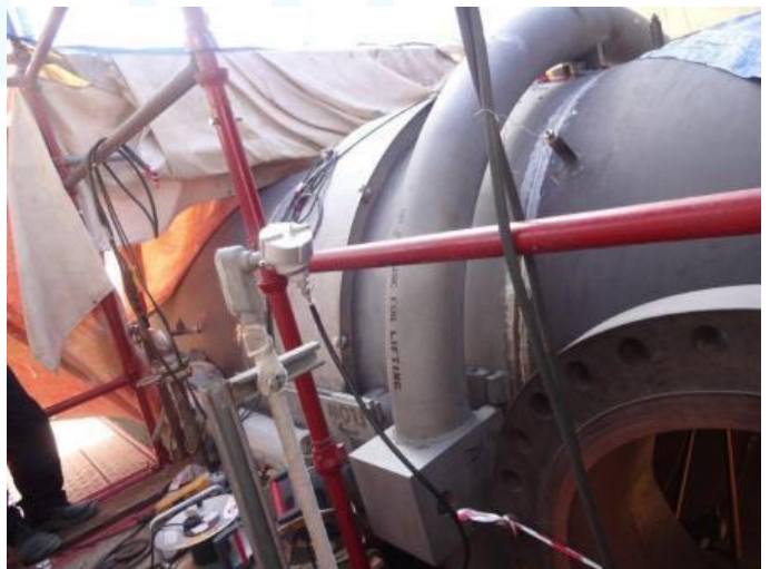
▼ Replacement of 78"Ø Air Line SS Pipeline Assembly (Expansion Joint Assembly: 2.5 tons). (5 th Floor)
