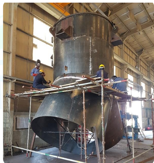
Emergency Vent Assembly Y
