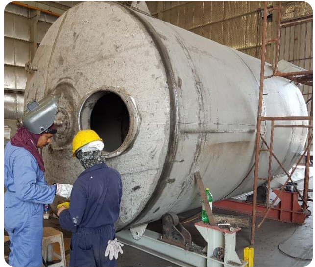
PHASE SEPERATION TANK (SS316)
