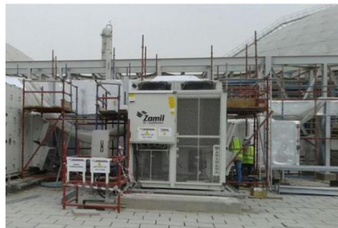
Aromatics MCC Building in SADARA Complex.
