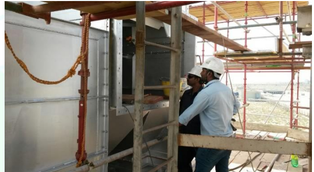
Out let duct connection
