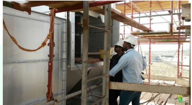
Out let duct connection
