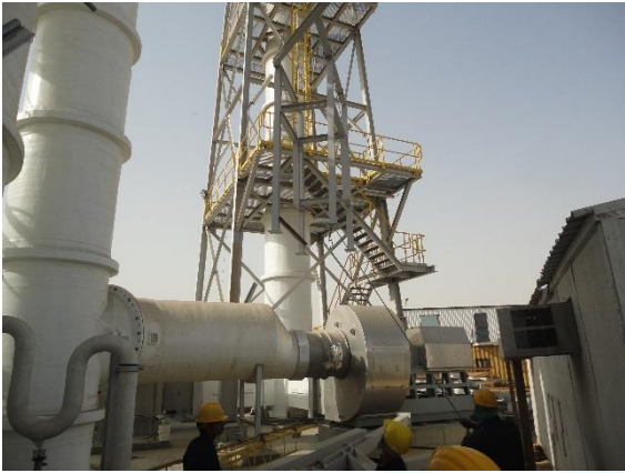
Scrubber to Stack Assembly
