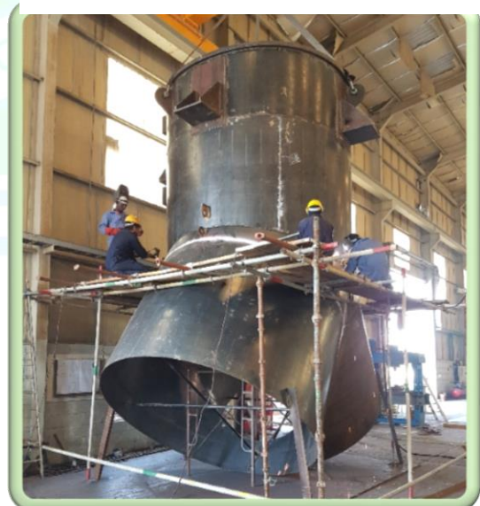
Emergency Vent Assembly Y
