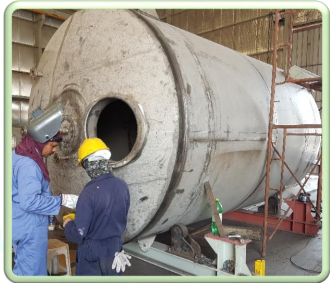
PHASE SEPERATION TANK (SS316)
