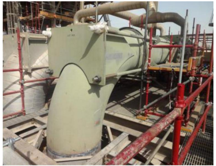
▲ Replacement of 42"Ø Air Line CS Pipeline Assembly along with the Expansion Joint Below. (4 th Floor)
